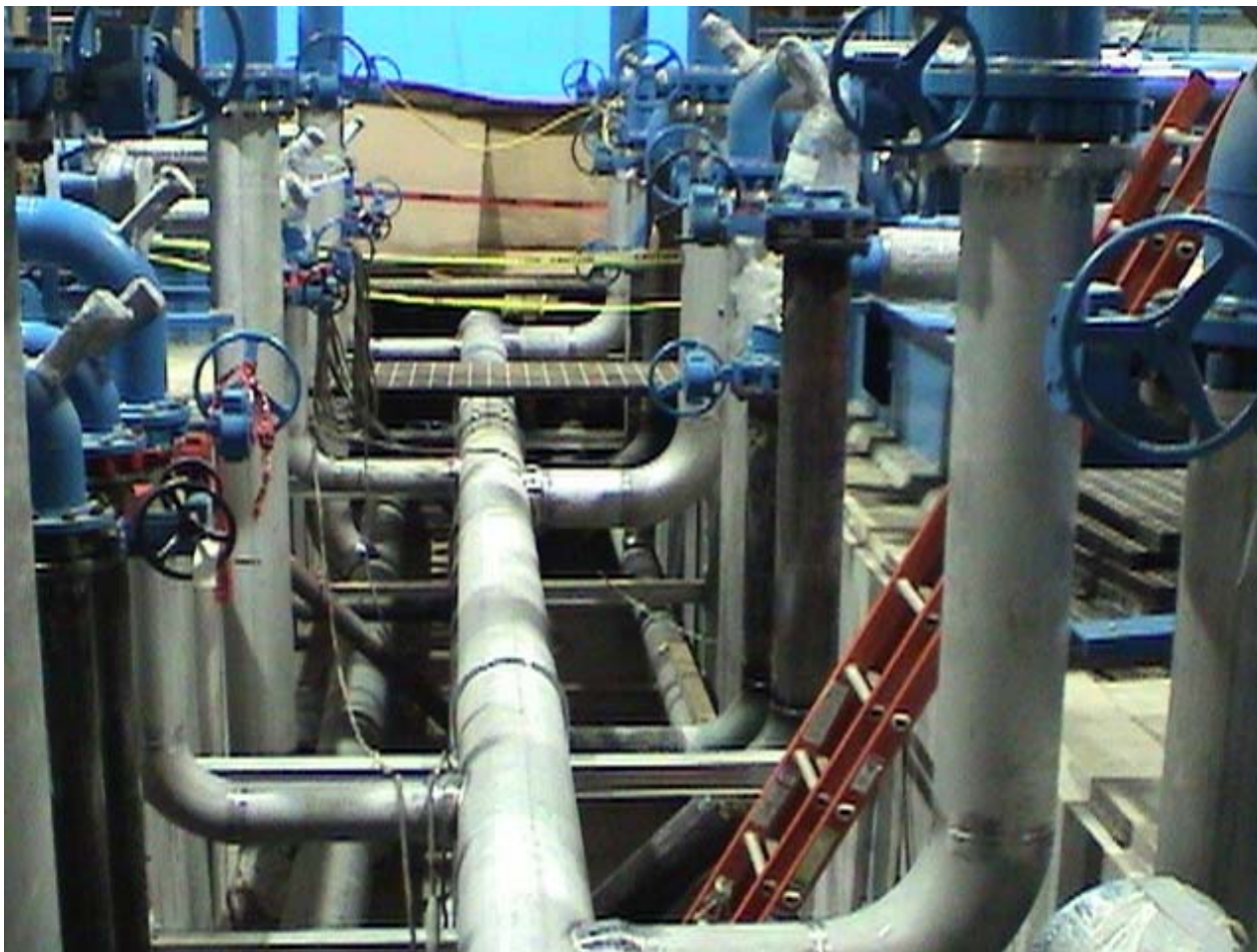
SNS Installation Shown
