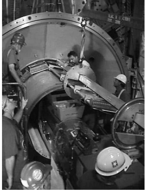
Figure 30. Installation of a bar box into the BABAR detector. Not seen in the figure is the cantilevered support arm which supports the installation fixture above the accelerator components.
