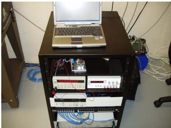
Data acquisition rack (S10)
