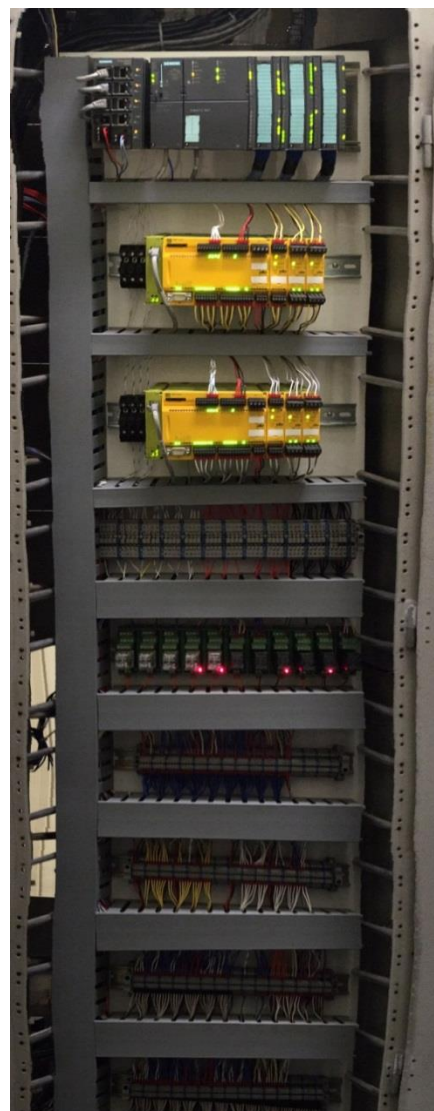
Figure 2: New Installation in repurposed racks.
